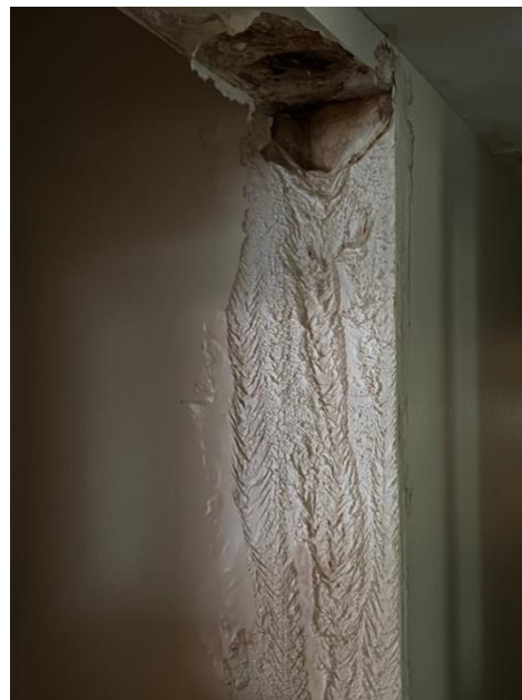
Figure 20: Water damage at door jamb
