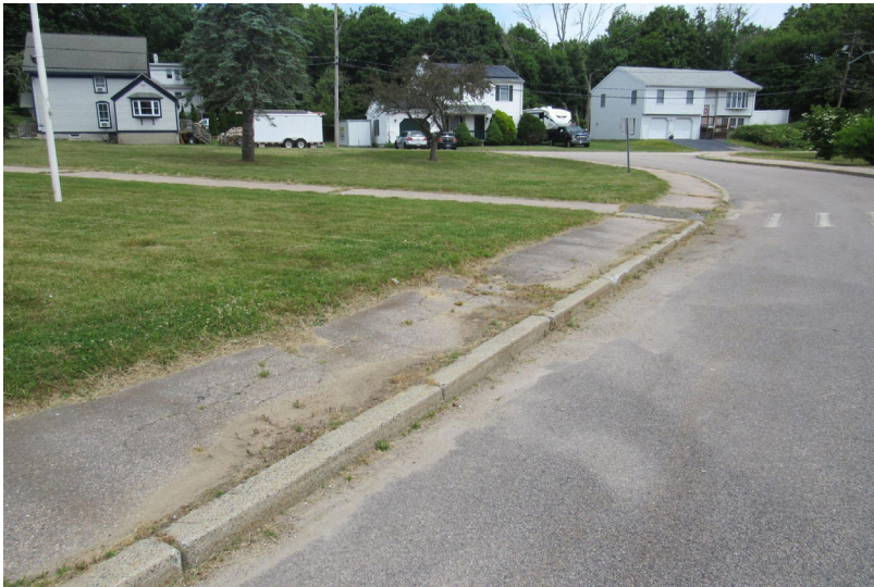
Additional view of asphalt-paved walkway deterioration as seen along front of building
