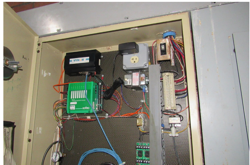
View of controls governing boiler plant performance
