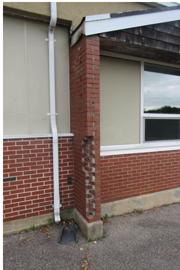
View of pronounced brick masonry deterioration (e.g., mortar loss, spalls, cracking) – observed at several locations
