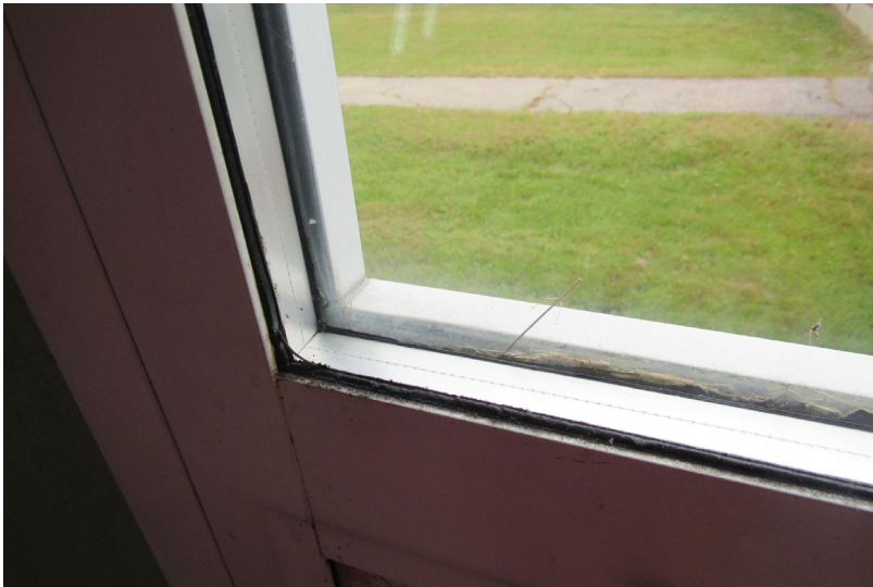
Exterior windows are predominantly aluminum-framed fixed and operable models – butyl bedding compound deteriorated at select locations
