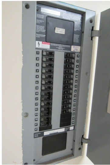
View of one of several electrical circuit breaker panels – mix of newer Siemens panels and possibly original panels
