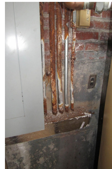
View of corroded electrical conduit present within central mechanical room
