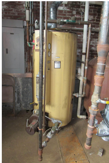
View of natural gas-fired domestic water heater facilitating domestic hot water (DHW) generation for building – 125-gallon storage capacity
