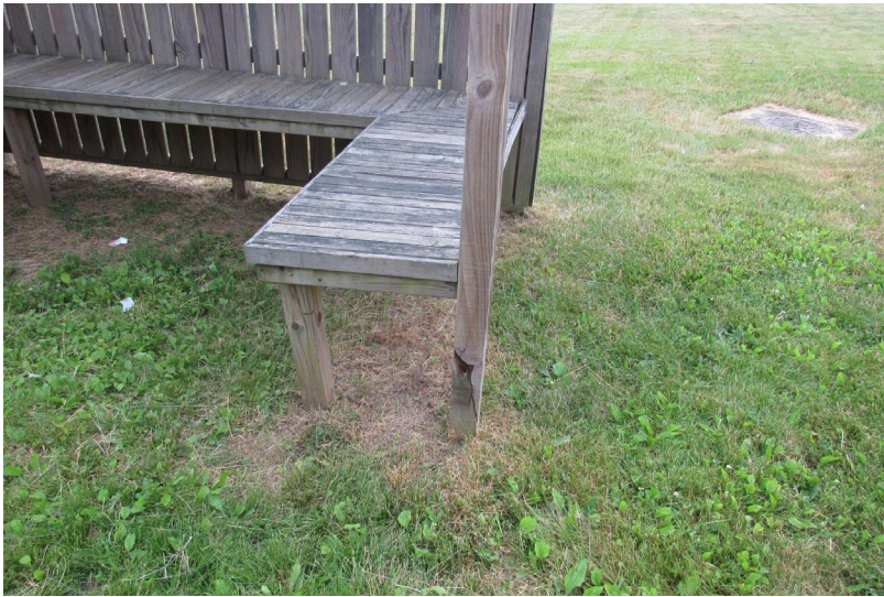
View of wood-framed bench structure exhibiting wear
