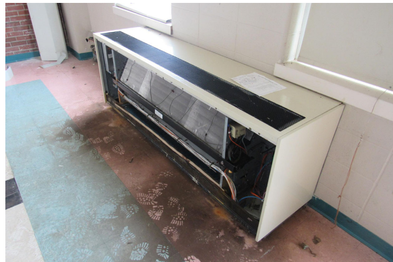
Several classrooms contain unit ventilators
