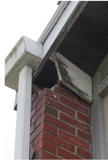
View of void/source of moisture and rodent ingress within building envelope as seen at north end
