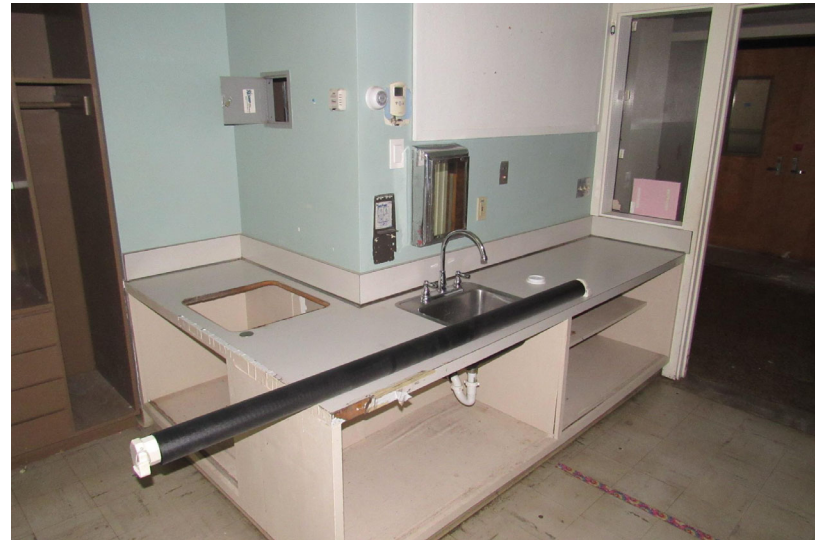
View of sample of classroom cabinetry – age related wear
