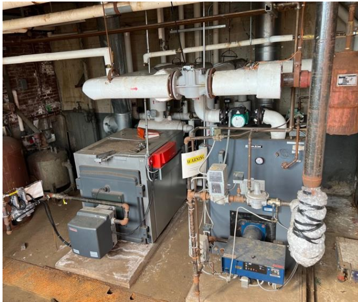
Figures 4 & 5: Boiler Room equipment
