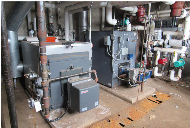
View of natural gas-fired boilers facilitating hydronic heat generation for building
