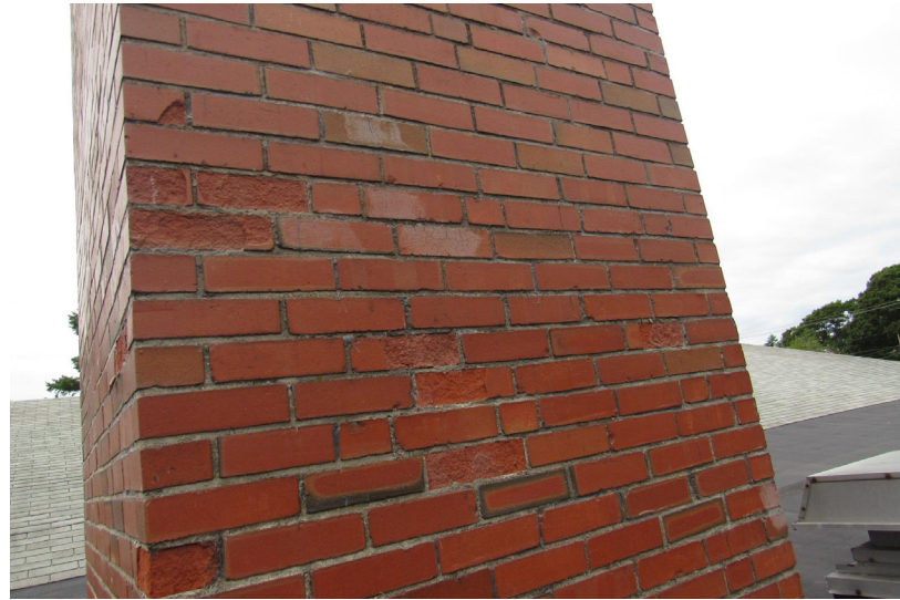
View of deteriorated brick masonry at chimney
