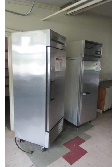
View of sample of commercial kitchen refrigeration equipment
