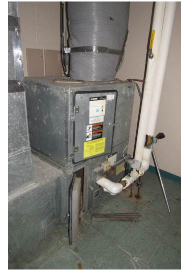
View of Trane fan coil unit (FCU) facilitating space heating distribution for select interior spaces
