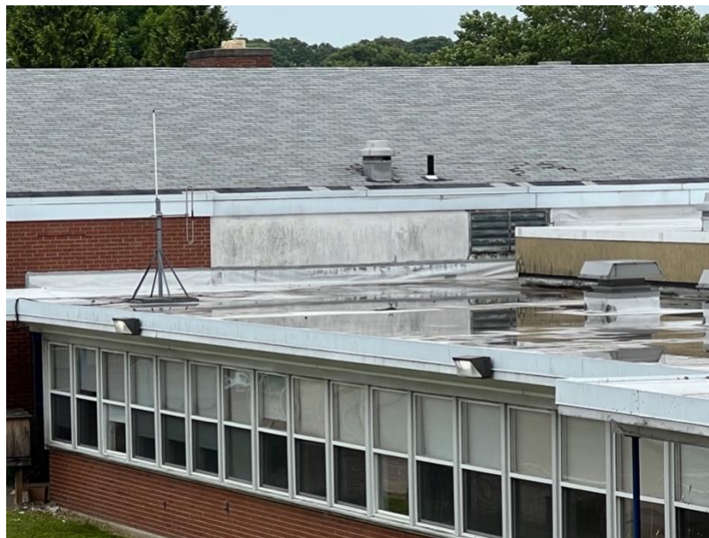
Figure 18: Tower Street School roof shows pooling
