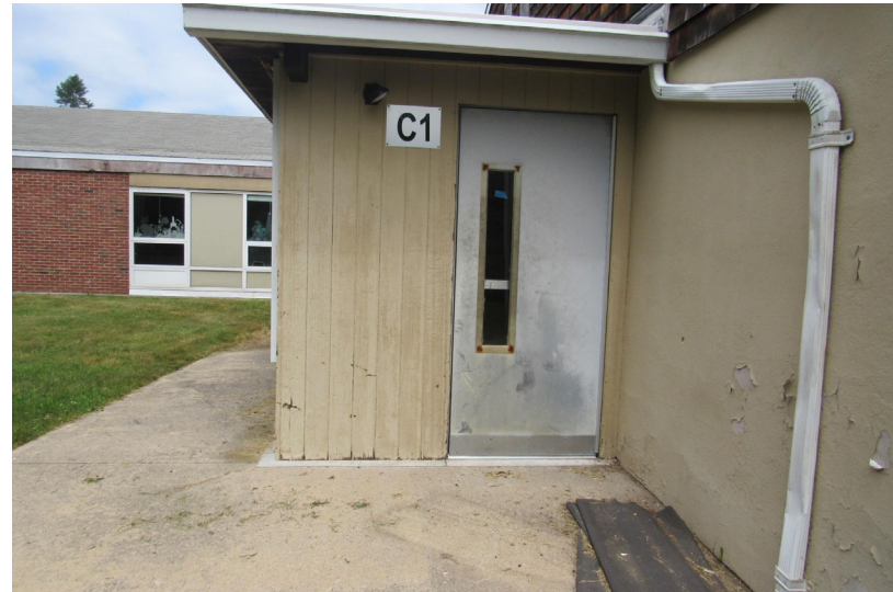
View of hollow metal emergency egress doorway exhibiting abrasions/wear
