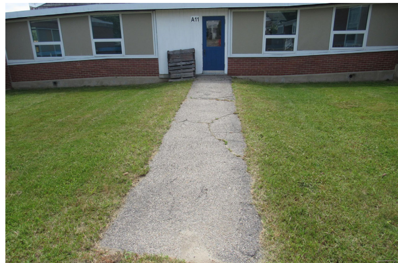
View of localized cracking within asphalt-paved walkway
