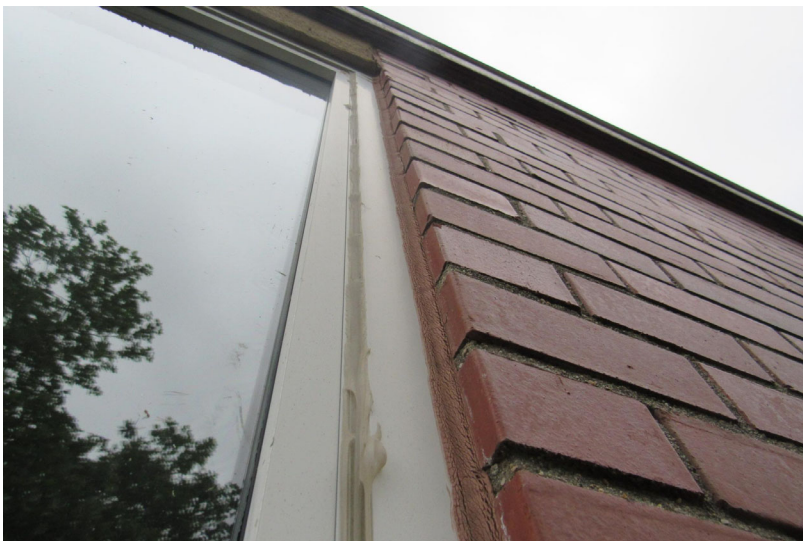
View of exterior window perimeter caulking conditions – note cohesive/adhesive failures
