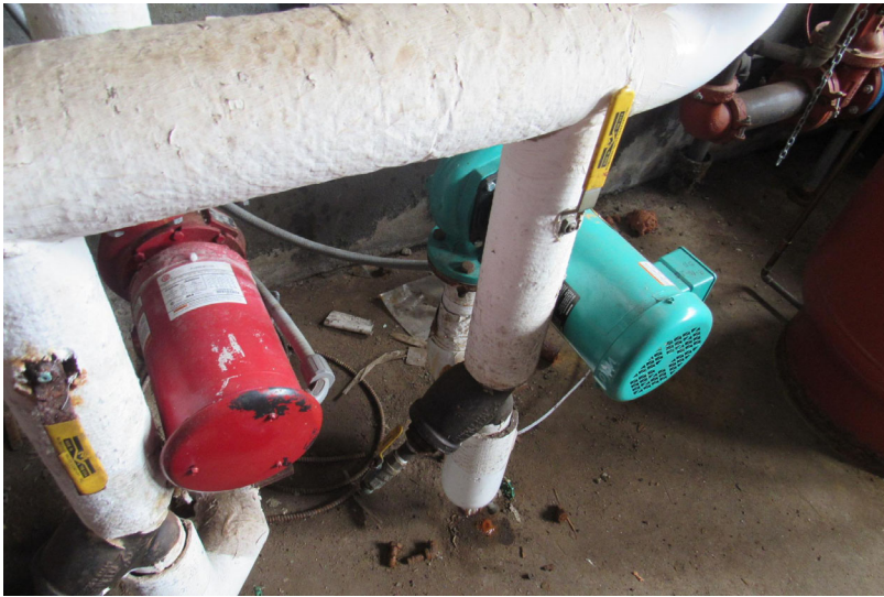
View of inline hydronic heat circulation pumps – 2 and 3-horsepower models
