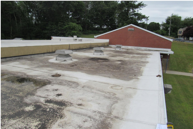
View of widespread staining and evidence of poor drainage on single-ply roof assembly – isolated membrane blisters also noted during site review (i.e., indication moisture has traveled beneath roof membrane)
