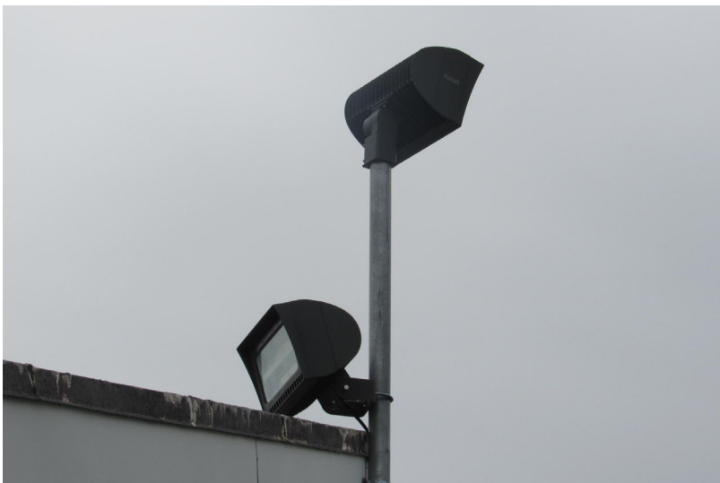
View of building-mounted light-emitting diode (LED) fixtures
