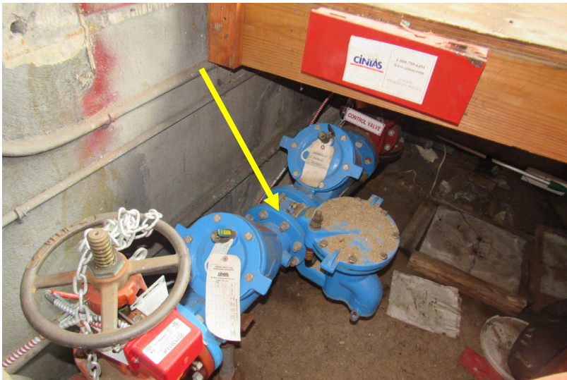
View of wet fire suppression system – note backflow preventer is in place
