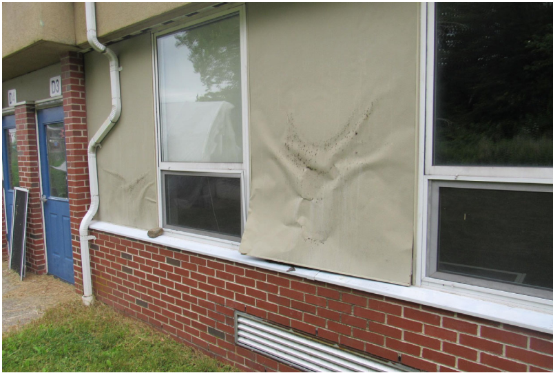
View of damaged metal paneling present at rear of building
