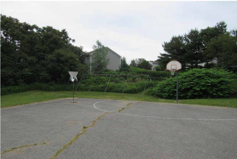
View of asphalt-paved basketball court present at south end of development – localized cracking noted
