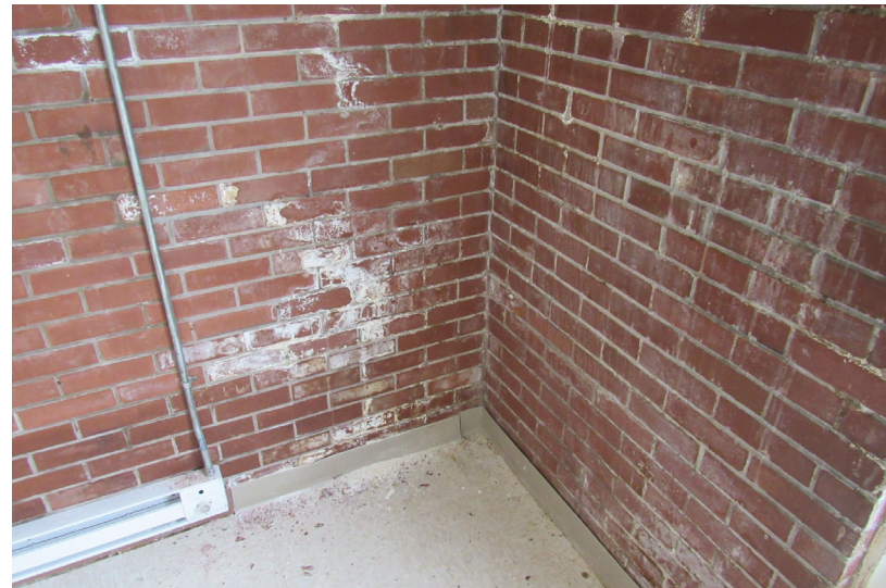
View of apparent efflorescence staining on interior brick masonry surfaces
