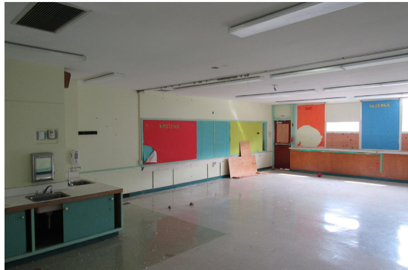
View of sample of classroom finishes – mix of painted wall and ceiling surfaces, suspended ceiling tile, vinyl composition tile (VCT), and suspected asbestos containing floor tile
