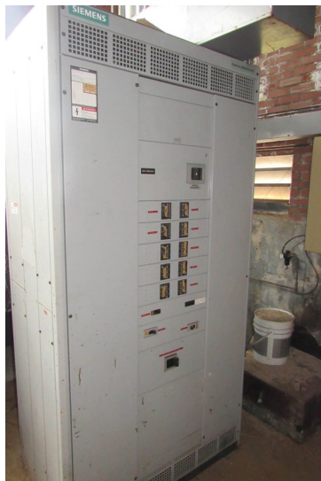
View of Siemens switchgear- 800 amps, 3 phase, 4 wire
