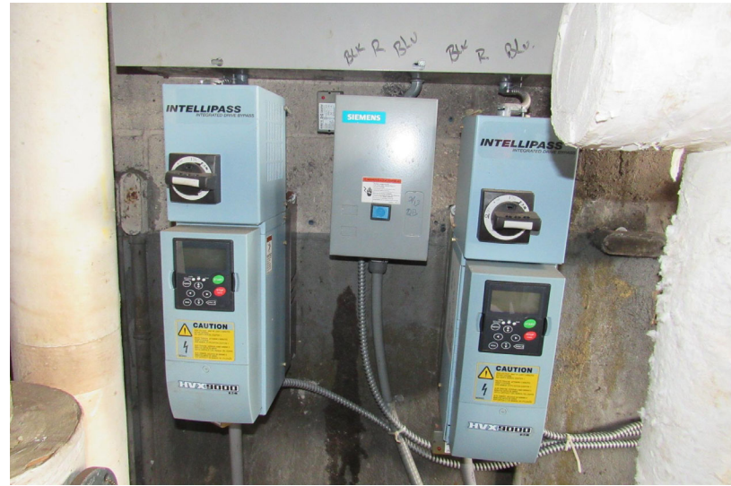
View of hydronic heat circulation pump variable frequency drive controllers
