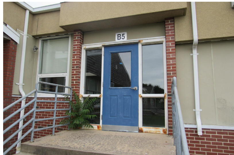
View of embossed two panel metal doorway and metal side lights exhibiting corrosion and age related wear
