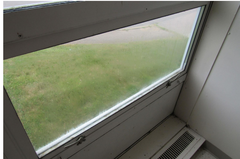
View of failed insulating glass unit (i.e., condensation formation between glass panes)
