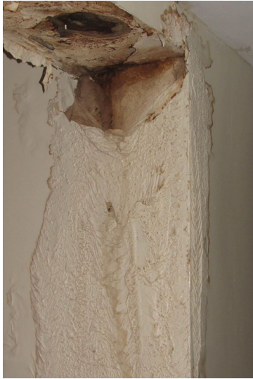
Localized moisture damaged finishes noted within interior spaces – potentially due to roof leakage or failed distribution piping
