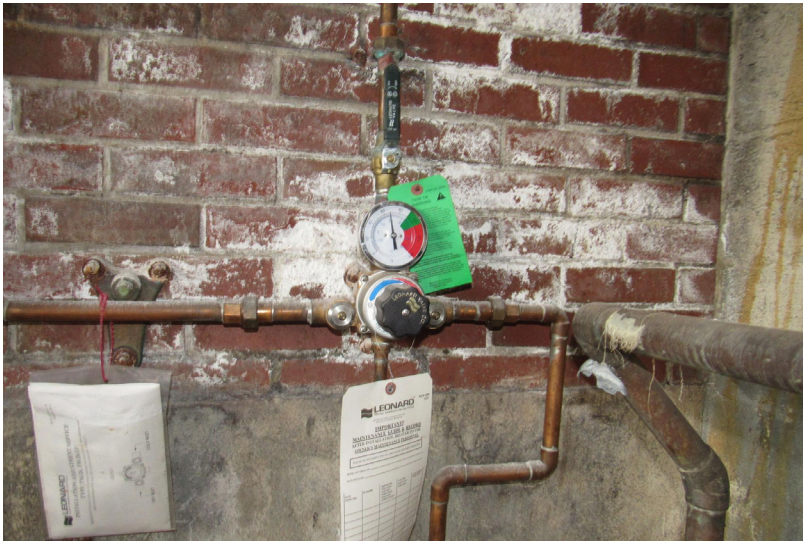
View of domestic hot water thermostatic mixing valve
