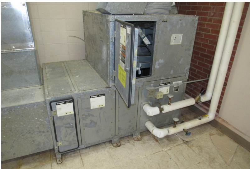
View of second Trane fan coil unit facilitating space heating distribution for select interior spaces
