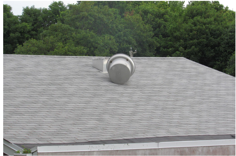
View of displaced rooftop-mounted powered exhauster present at west end of building
