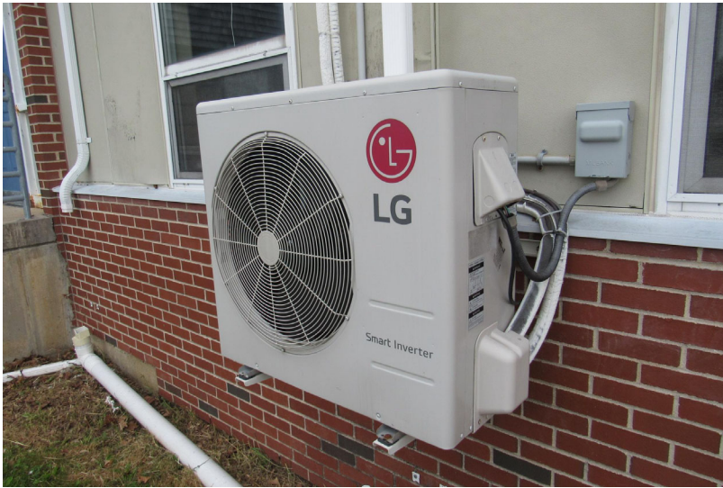
View of LG ductless mini-split system air conditioner
