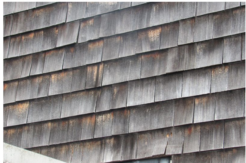
View of wood shake siding exhibiting age related wear
