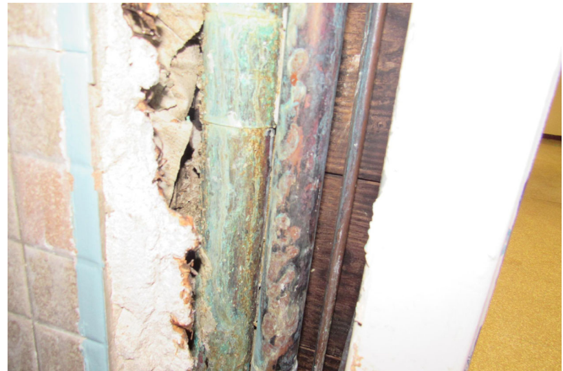
View of sample of distribution piping exhibiting oxidation/wear
