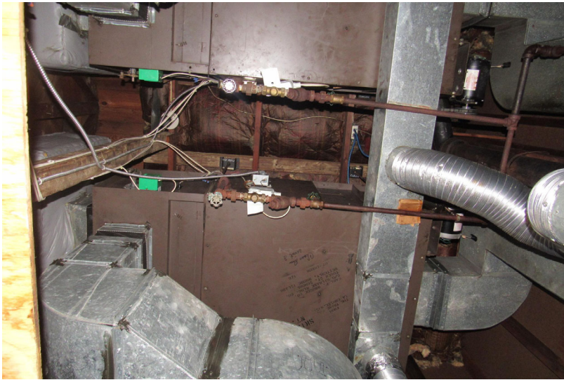
View of one of several interior heating and ventilation units serving rear (i.e., south end) classrooms
