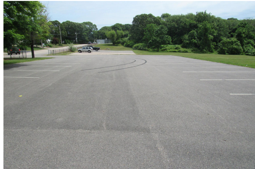
Additional view of asphalt-paved surface parking area conditions – no widespread cracking, depressions, or evidence of fatigue observed
