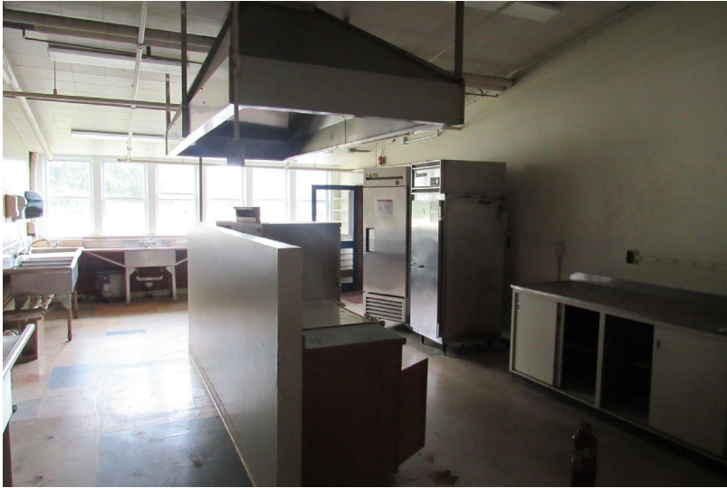
View of commercial kitchen finishes and equipment
