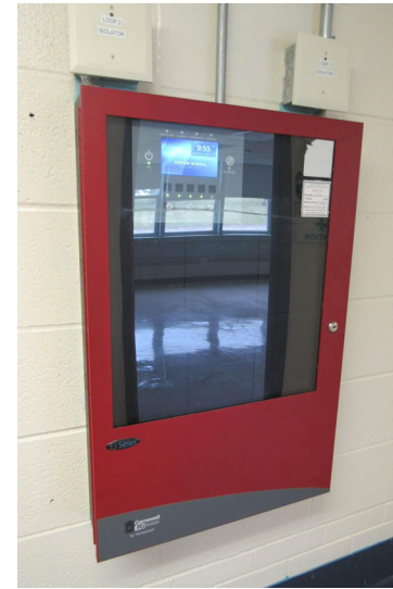
View of fire alarm control panel monitoring hardwired end devices
