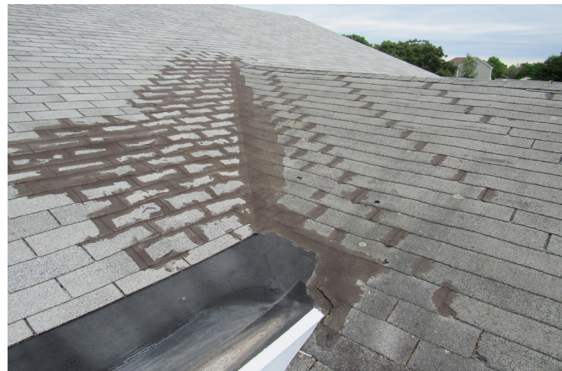
View of evidence of previous mastic-type repairs to roof valley and shingles
