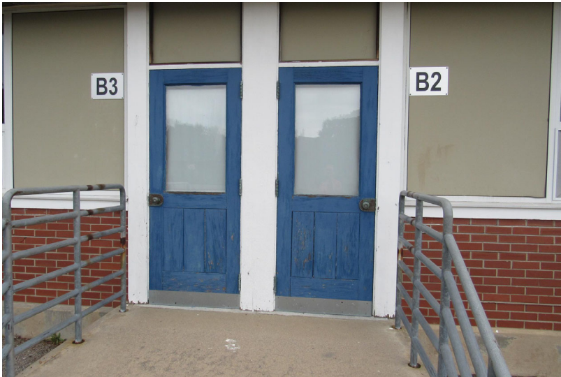
View of solid core wood emergency egress doors exhibiting age related wear
