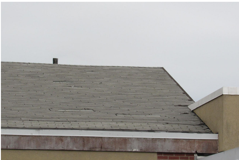
View of displaced three-tab asphalt roof shingles – observed at several locations
