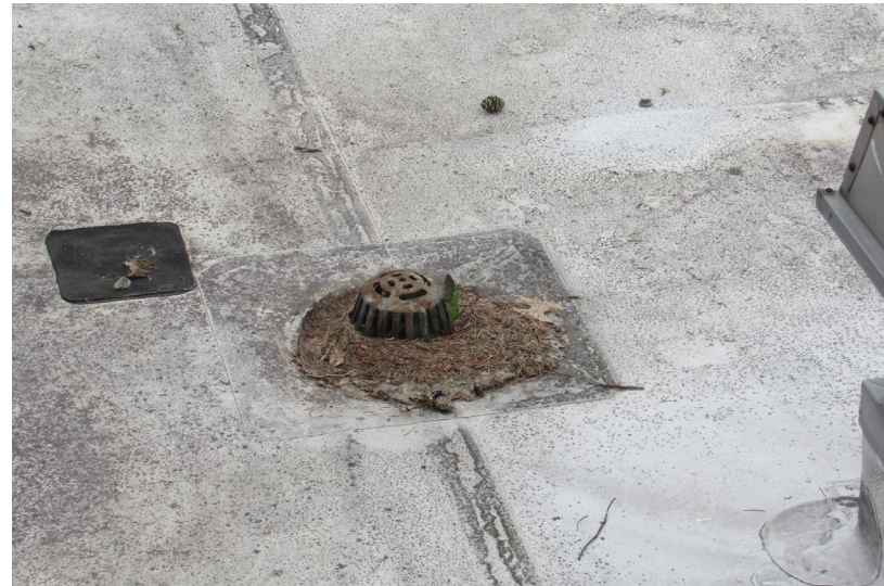
View of accumulated vegetation around strainer dome restricting adequate roof drainage
