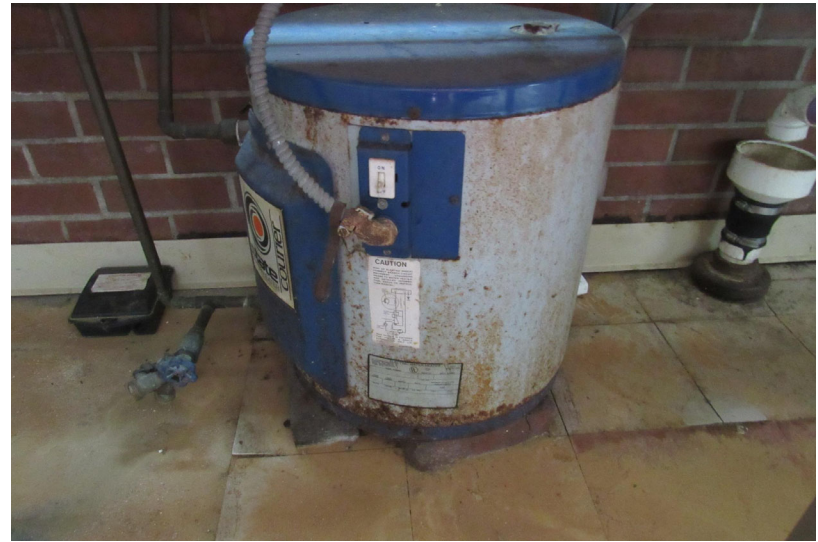
View of electric domestic water heater serving commercial kitchen equipment
