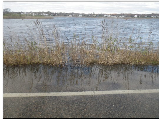
WETLAND OVERTOPPING ROADWAY: NORTH SIDE
